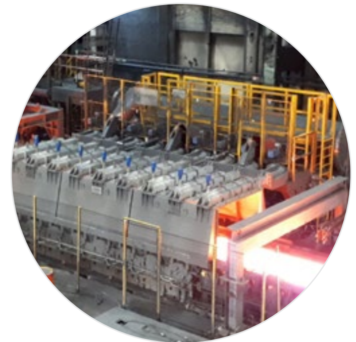
Transfer bar cooling unit installed at TATA Steel, Port Talbot
