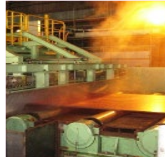
MULPIC at Baosteel Zhanjiang Iron & Steel, Zhanjiang, China
